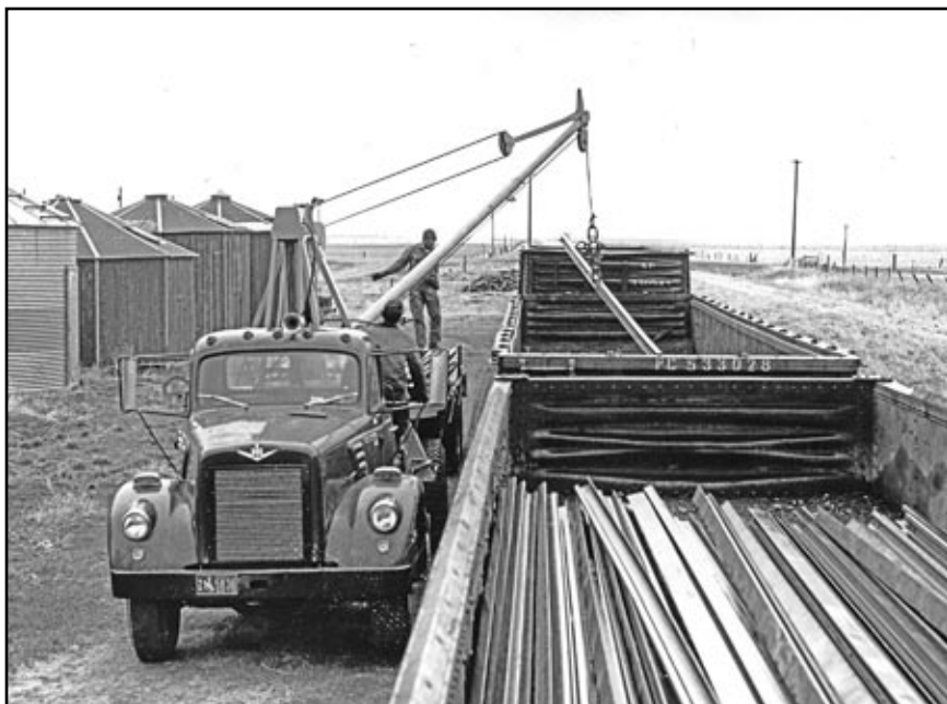
Loading salvaged rail into gondola cars at Carpenter, Wyoming, on April 12, 1970. – Photo © James L Ehernberger.
