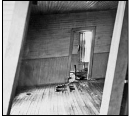
The interior of the boarding house, already leaning away from the tracks but still standing on July 31, 1951. – Photo © Bill Abbott.
