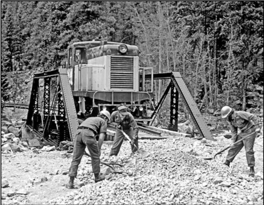
SeaBees do grading work at the Georgetown Loop Pin Truss bridge. – Photo © Bill Robie.
