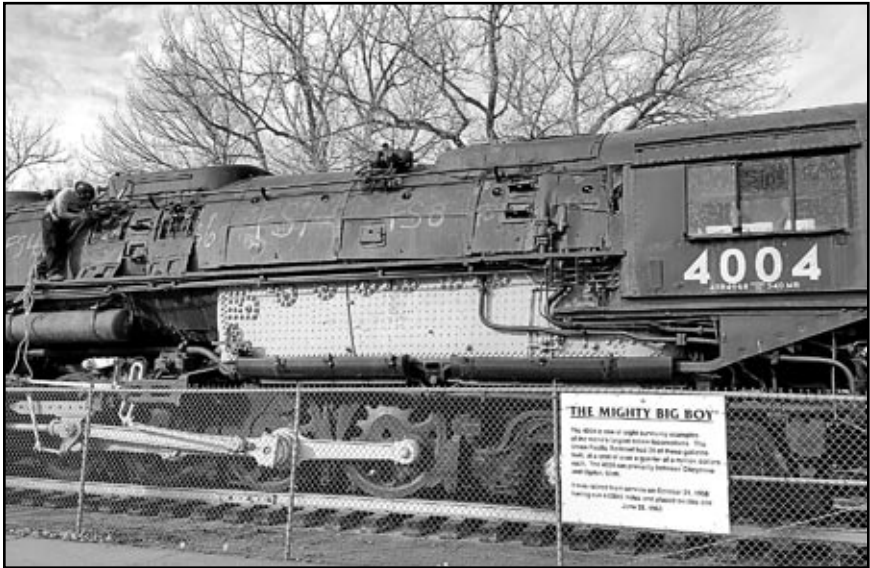
Preparation work in advance of asbestos removal on UP “Big Boy” 4004 at Holliday Park in Cheyenne, Wyoming. – Photo © 2018 Dave Schaaf.
