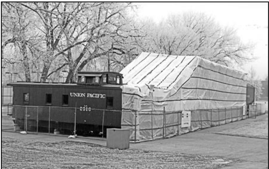
UP “Big Boy” 4004 is encapsulated in preparation for asbestos removal on February 9, 2018. The UP caboose (on a frame, without trucks) is privately owned and is used as a warming shelter and a place for changing in and out of proper safety apparel required for asbestos removal workers.
